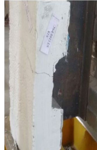
Fig. 26. Crack pattern in slab 'PET2'
