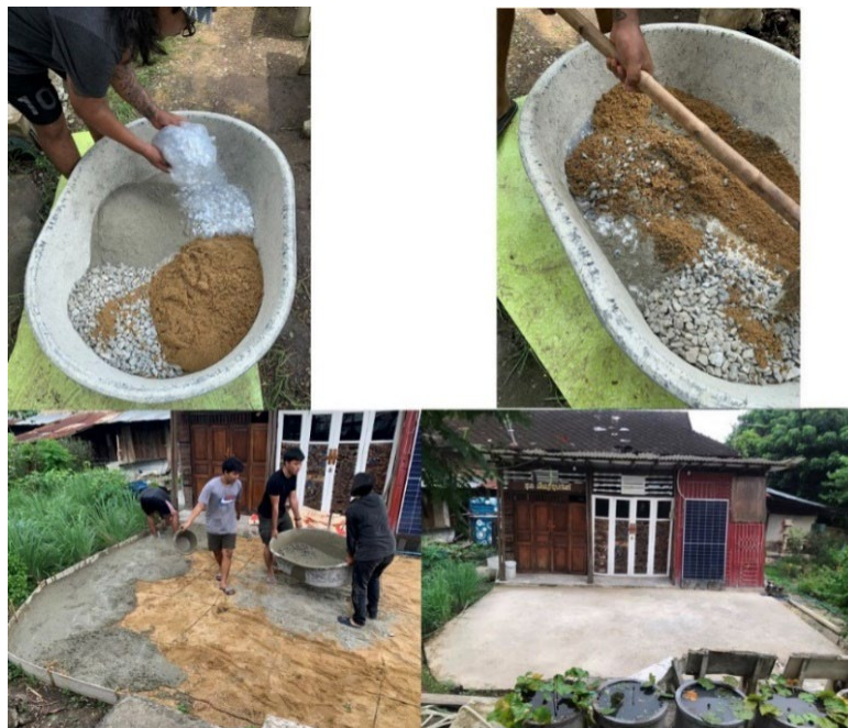
Fig. 8. Construction of a multi-purpose concrete courtyard floor of Minburi Upatham Community, Minburi District, Bangkok, Thailand by ECPS
