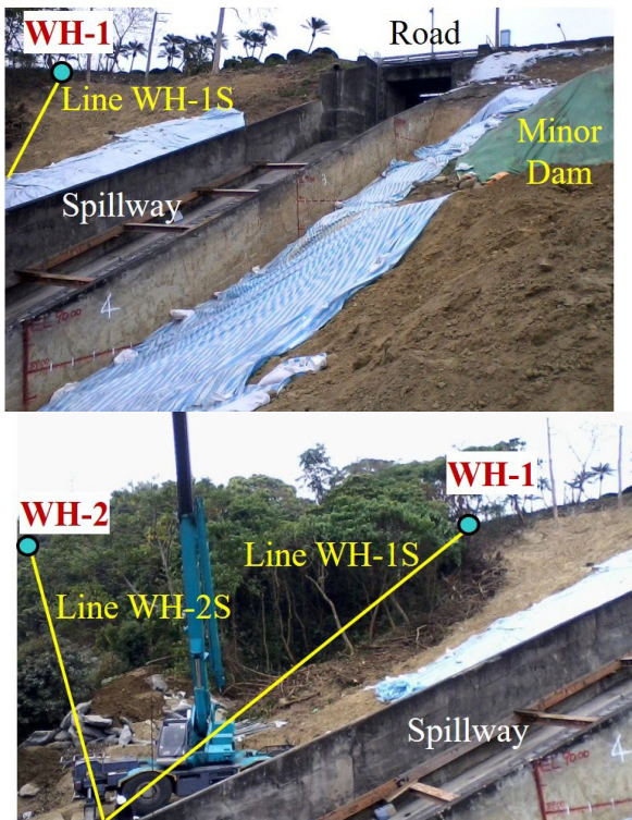
Fig. 4. Surface sliding along the damaged spillway
